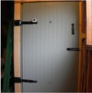
Door. Note huge hinges and internal temp monitor.
